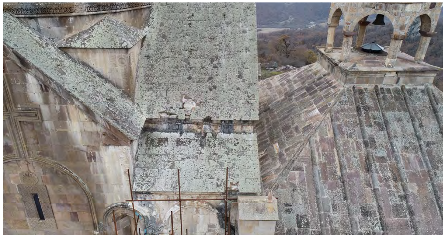
Fig. 11. Deteriorations on the northern roof's pitch on the church's western arm (Iconem 2020)
