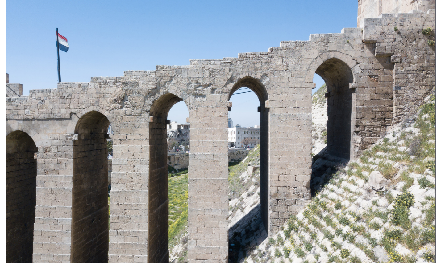
Bridge linking the outer gate (Madkhal Qal'a Halab) to the inner gate of The Citadel
